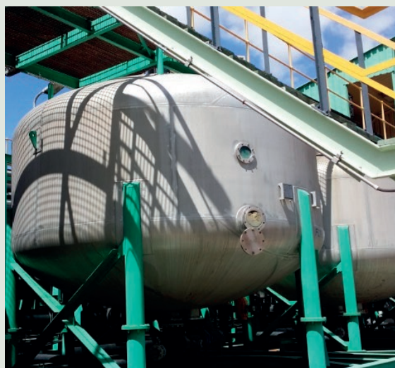
Figure 5: Choked electrolyte filter due to a gypsum-silica precipitate.
